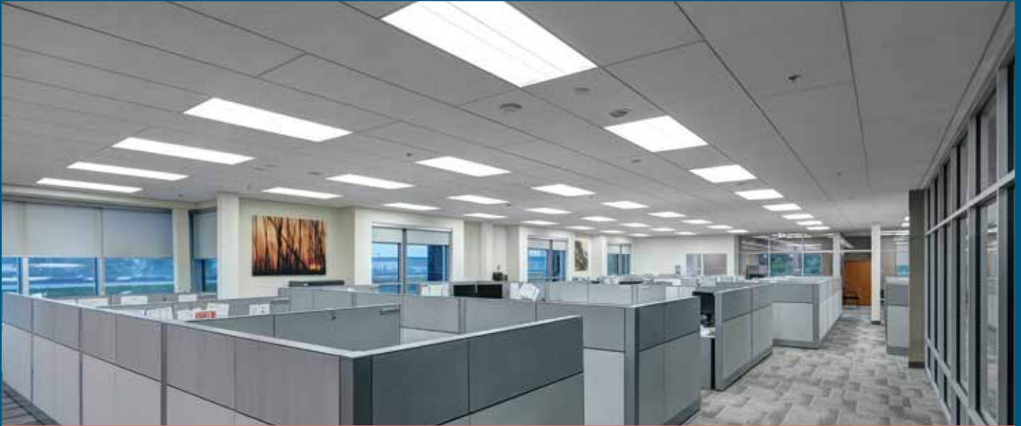
The open office areas showcase ROCKFON Sonar stone wool 2-by-8-foot ceiling panels with an exposed grid in a staggered pattern for visual interest and to easily accommodate the recessed lighting.
