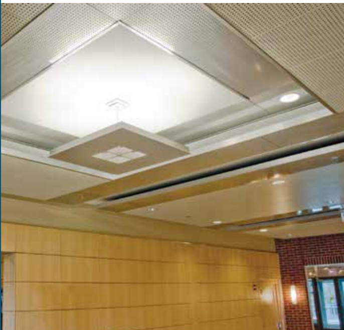
Clouds within clouds. In addition to adapting Chicago Metallic's suspension system to the center's design, each of the 34 different ceiling panel sizes, used throughout the center, needed to be precisely engineered to install perfectly out of the box.
